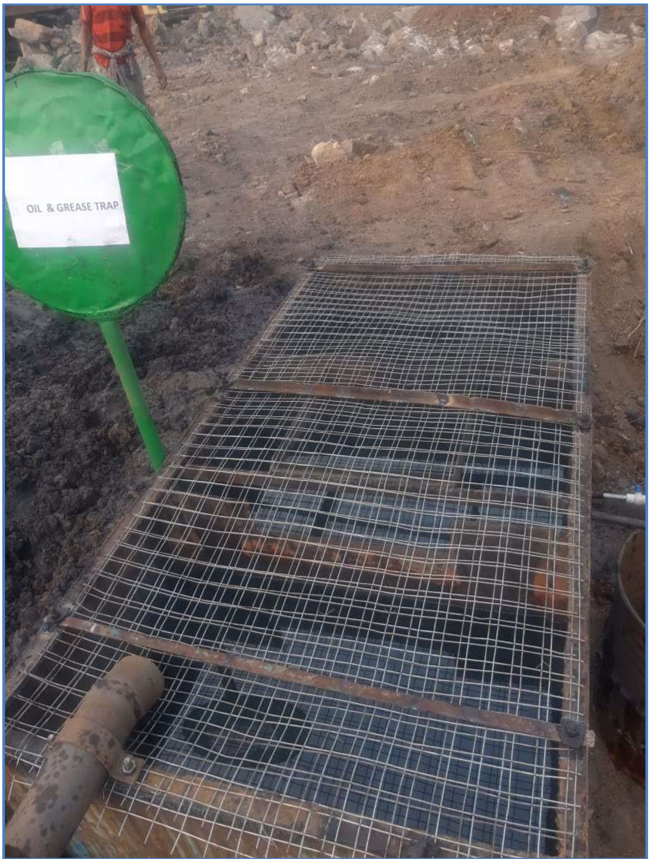
Picture 5 – Oil & Grease Trap
