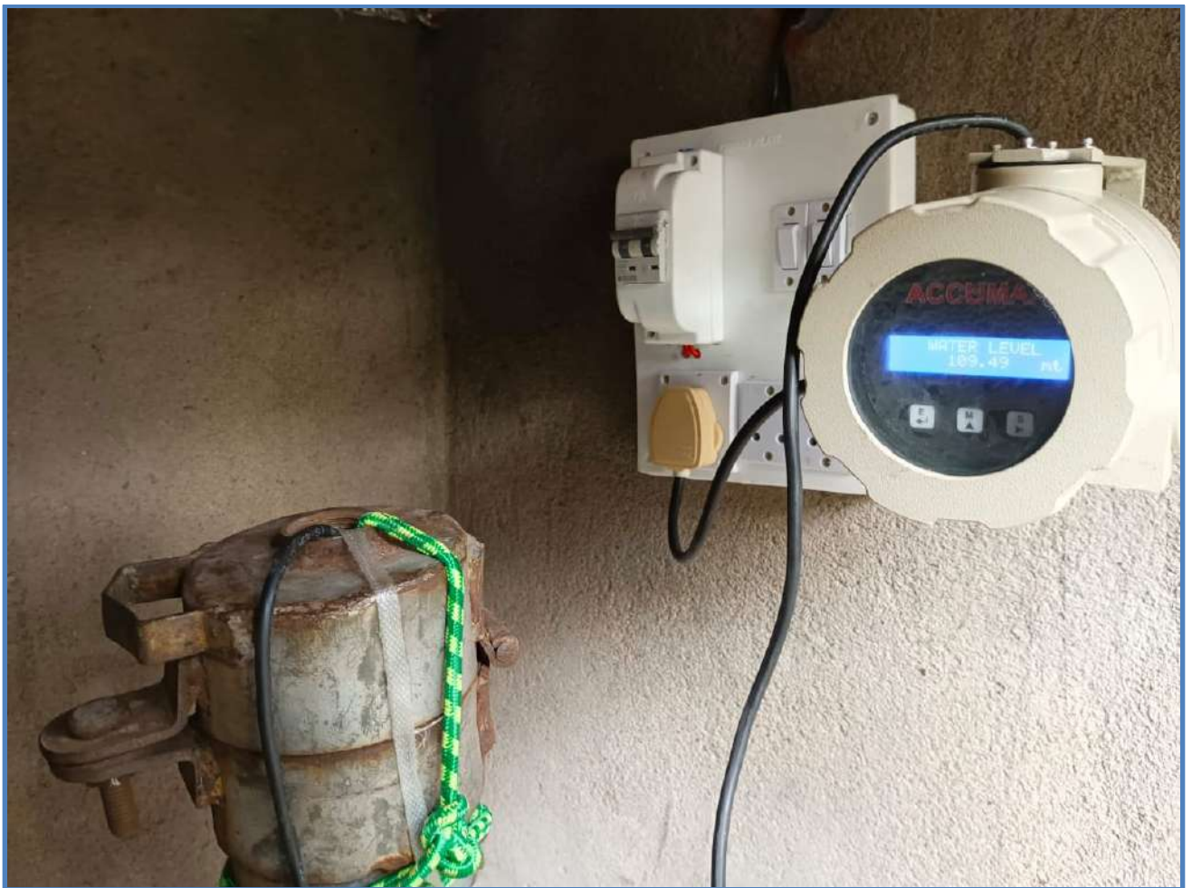
Picture 7 – Piezometric well with DWLR
